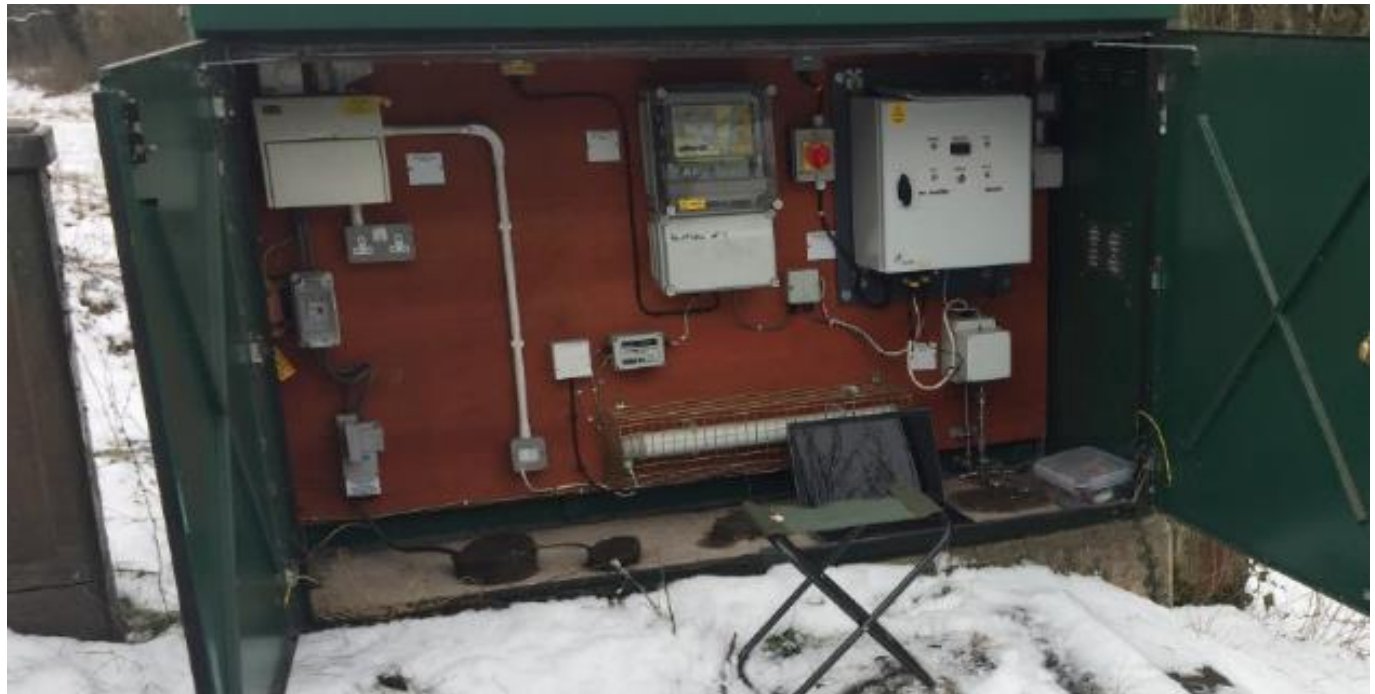
Unit installed in a cabinet. There are 6 of these cabinets on the industrial estate and include heating system, lighting protection and connection to the telemetry system.
